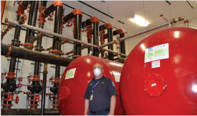
Multiple foam-water deluge systems protecting the entire hangar floor space. Each deluge system protected an area over 9,000 square feet each.
