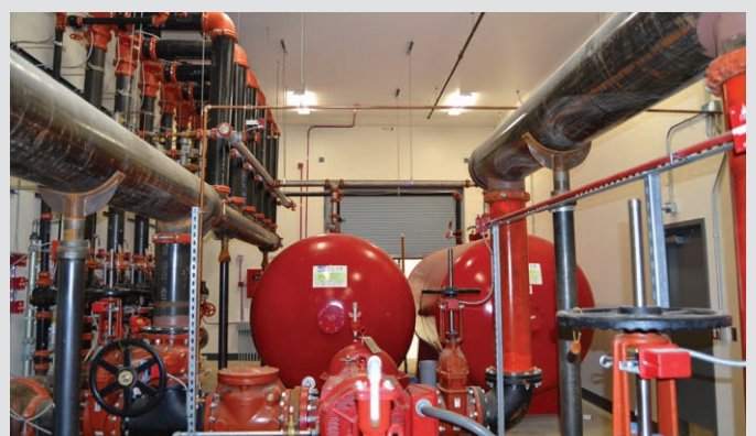
Two 2,600 gallon horizontal bladder tanks containing a total of 5,200 gallons of SOLBERG RE-HEALING RF3 3% Fluorine-free foam.
